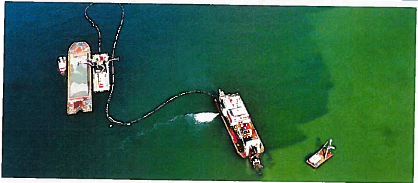
Dredger from Weeks Marine dredging a channel off Treasure Island, Florida (Photo: Dredging Contractors of America)
